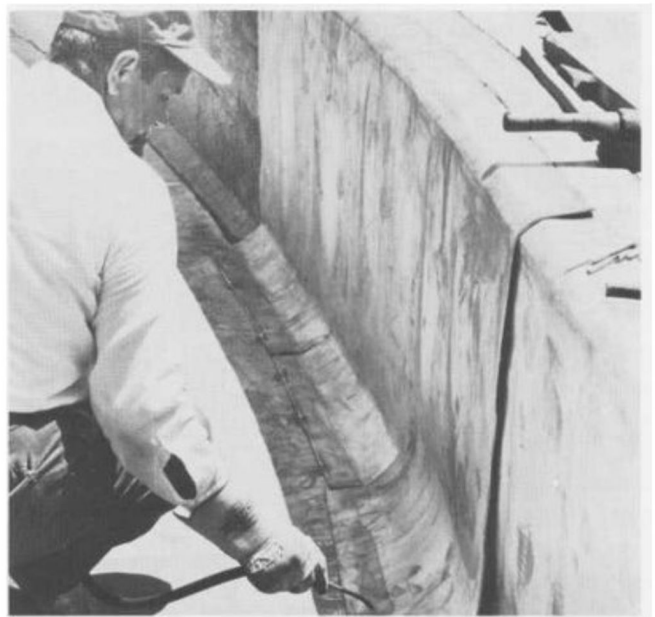
Reflecting pools and decorative fountains make extensive use of sheet lead waterproofing. The sheets on the sides are formed to follow the cant profile, then burned (welded) and flashed to other sheets to complete the waterproofing integrity.
